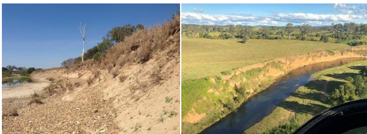
Figure 1. Stream bank erosion along the O'Connell River (left) and Mary River (right).
